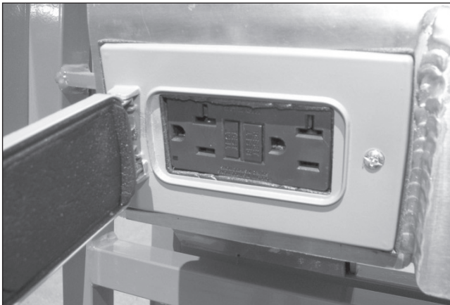
Figure 9.6 – Electrical Power Outlet
